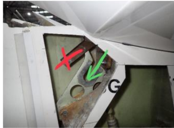
Disconnected elevator control
